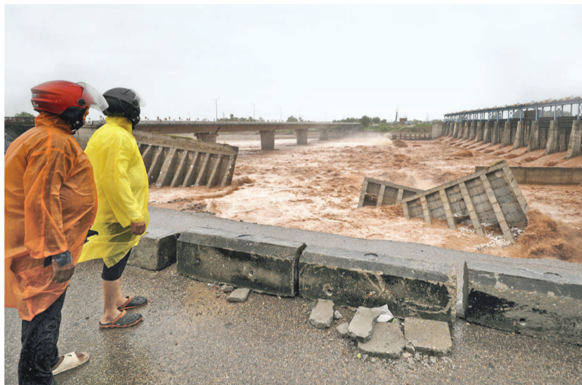
People protect themselves with raincoats while looking at the damaged remains of the 4th Tawi Bridge, after rain continues to lash parts of the city, in Jammu. PTI
